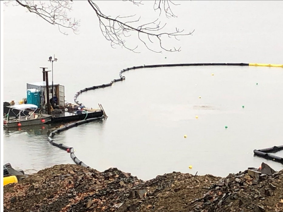
View from Getchell Property, Durham, NH showing diver barge (left), bottom-founded turbidity barrier, northern cable (yellow buoys) and center cable (green buoys). Surface indication (bubbles) of diver working on northern cable.
